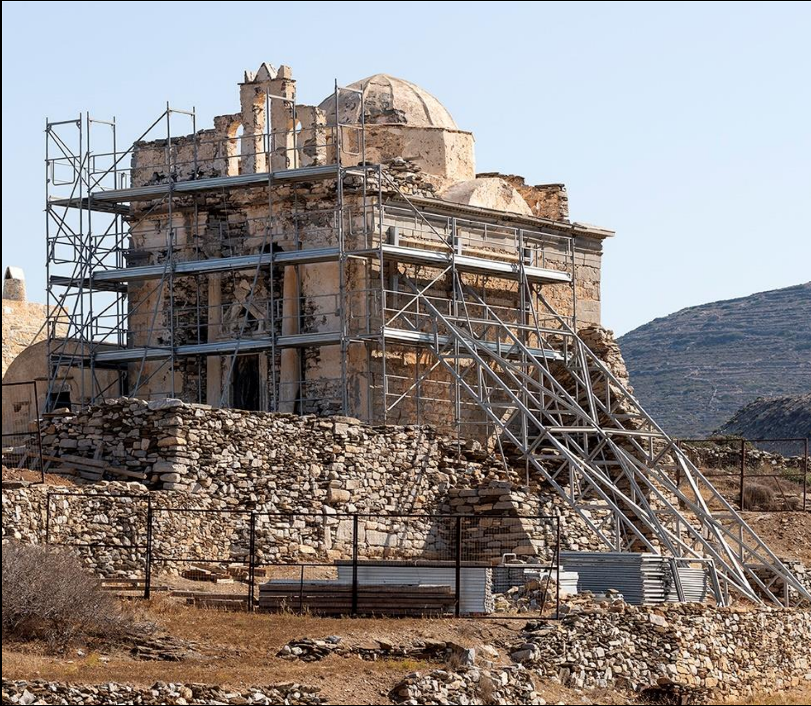
During the restoration project – exterior scaffolding and metal supporting of the outward inclined south wall
